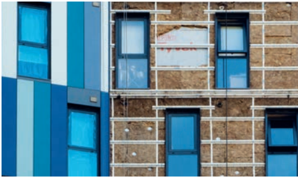
Left: Cladding in the process of being removed from a student accommodation building
