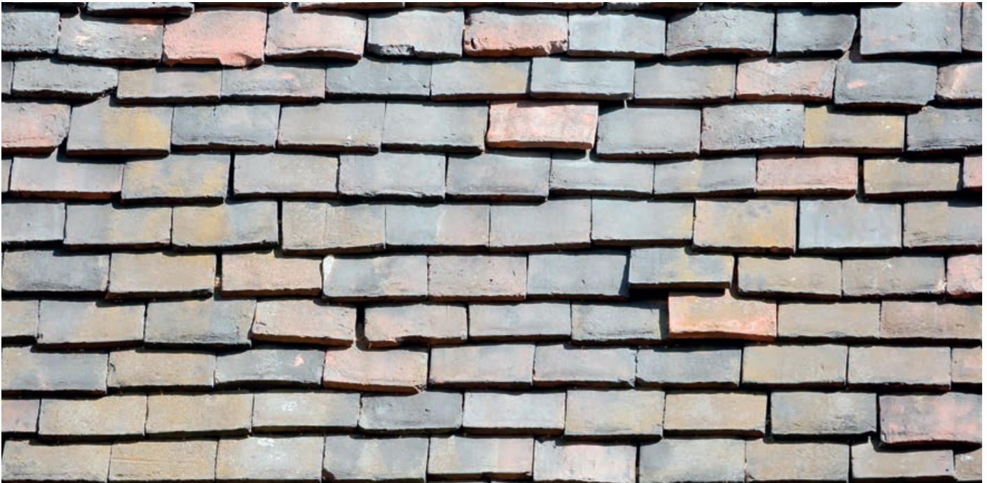
Above: Old roofs may be unsuitable for PV installation
